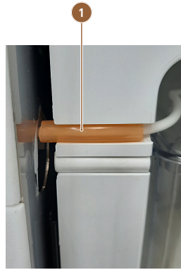
Fig. 50: Milk hose in cooling unit
